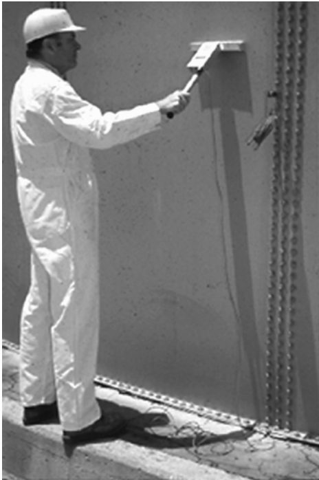
Figure 35. Using a low-voltage wet sponge holiday detector to locate discontinuities in non-conductive coatings applied to conductive metal substrates.
