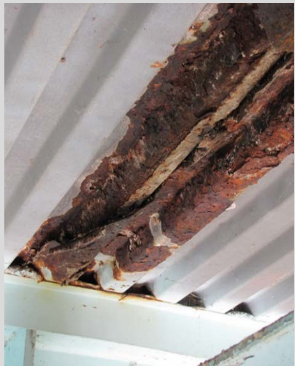
Condition State 3 Steel stay-in-place forms on underside of concrete deck rusted through
