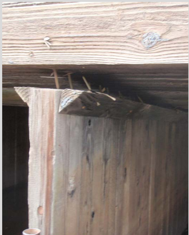
Condition State 4 Separation (connection failure) between wall and ceiling on a timber box culvert
