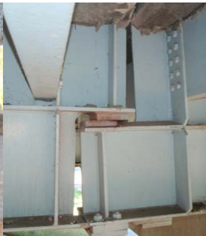
Misaligned hinge bearing
