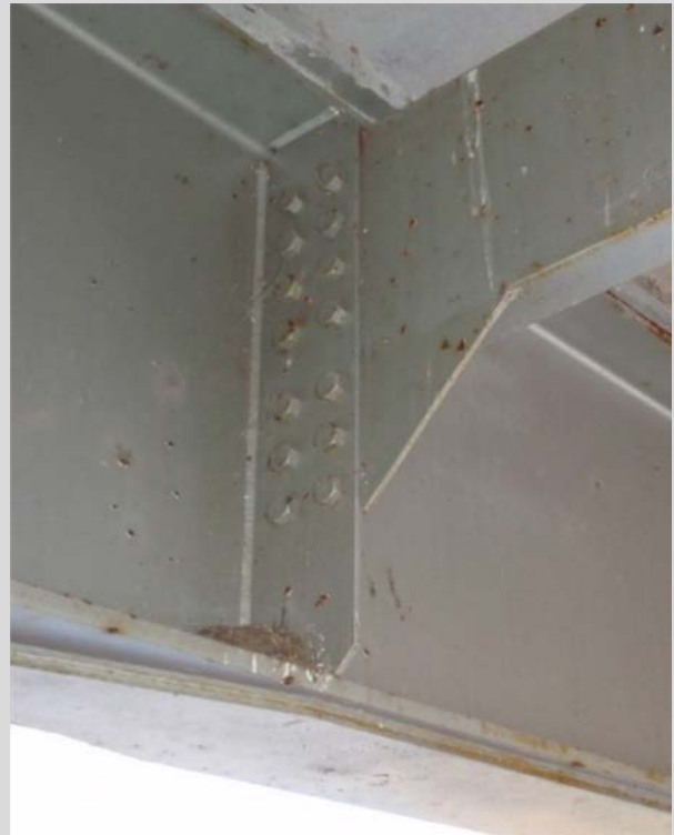
Condition State 2 Minor paint failure (Isolated – less than 3%)
