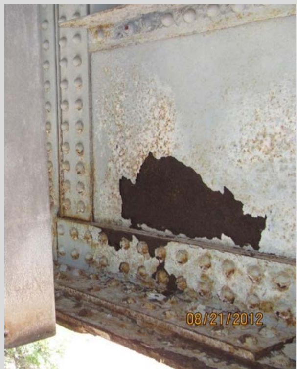
Condition State 4 Paint system failure (exposed steel)
