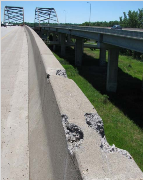
Condition State 3 Spalling along the top of a concrete J-rail
