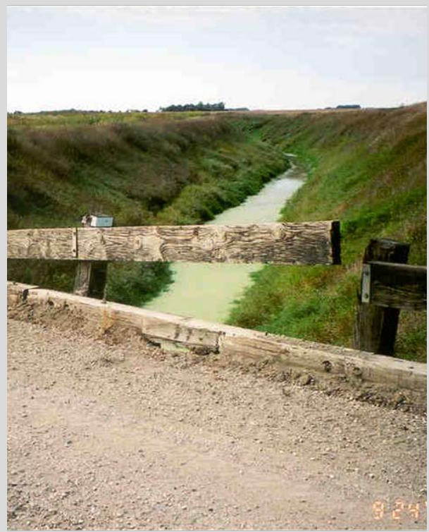
Condition State 4 Timber rail beam detached from posts
