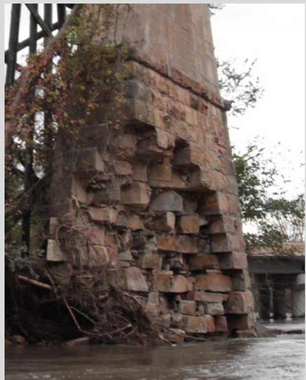
Condition State 4 Masonry pier wall severely damaged by scour
