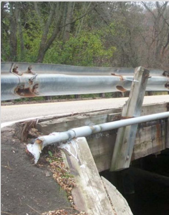
Condition State 4 Timber rail post missing (adjacent post is severely damaged)
