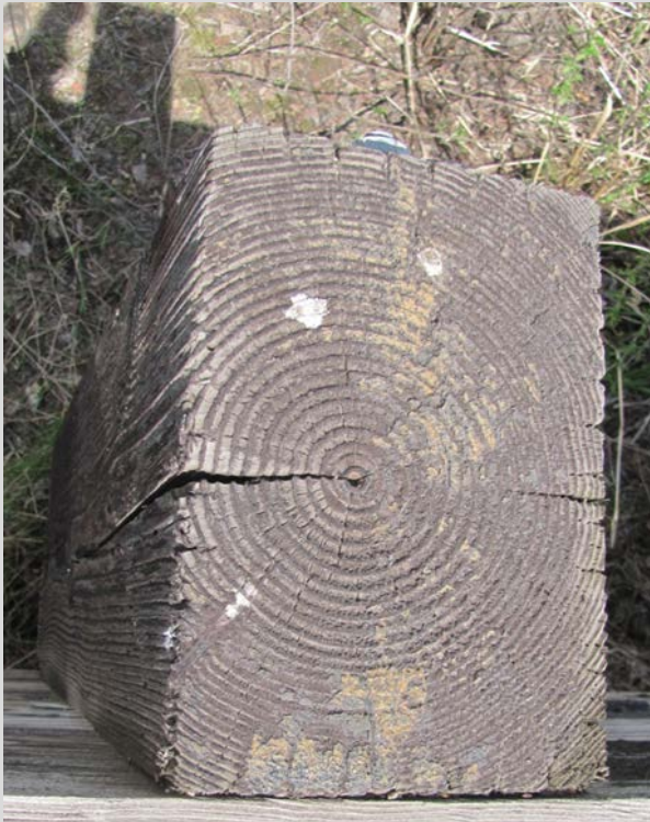
Condition State 2 Checks in a timber rail post
