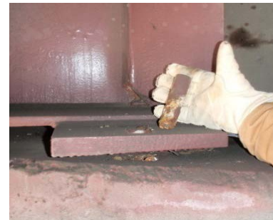
Anchor bolt failure on a fixed bearing
