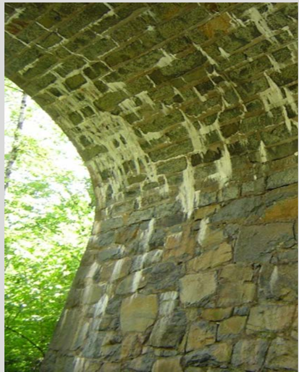
Condition State 3 Leaching through joints on a masonry arch
