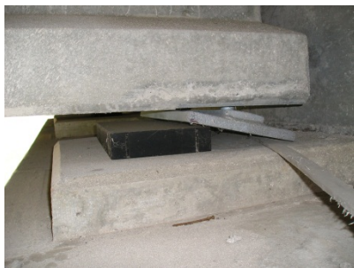
Severe malfunction of an elastomeric bearing
