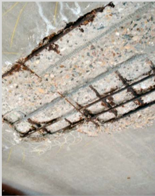
Condition State 3 Spalling (deeper than 1") with exposed and corroded rebar on the underside of a concrete deck
