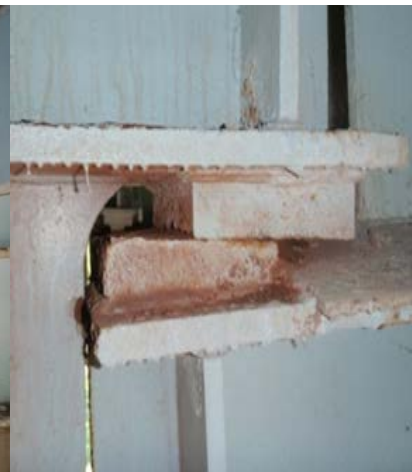
Hinge bearing in full expansion (beam ends contacting)
