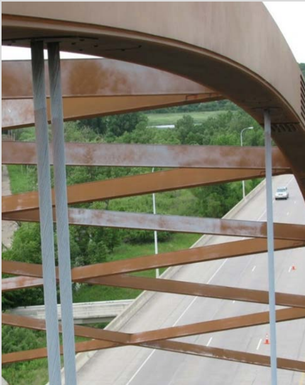
Condition State 2 Chalking paint on steel arch bracing members
