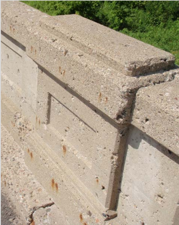
Condition State 2 Scale and pot-outs on a solid concrete parapet railing
