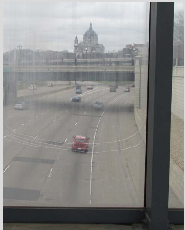
Condition State 3 Cracks in a transparent panel
