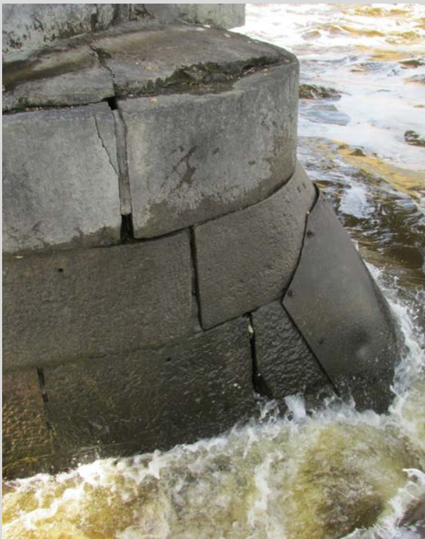
Condition State 3 Extensive mortar loss on a masonry arch
