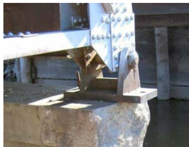
Fixed pin truss bearing with severe loss of bearing area
