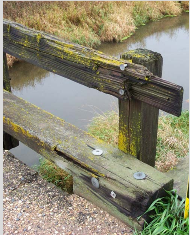
Condition State 3 Significant decay on a timber rail beam
