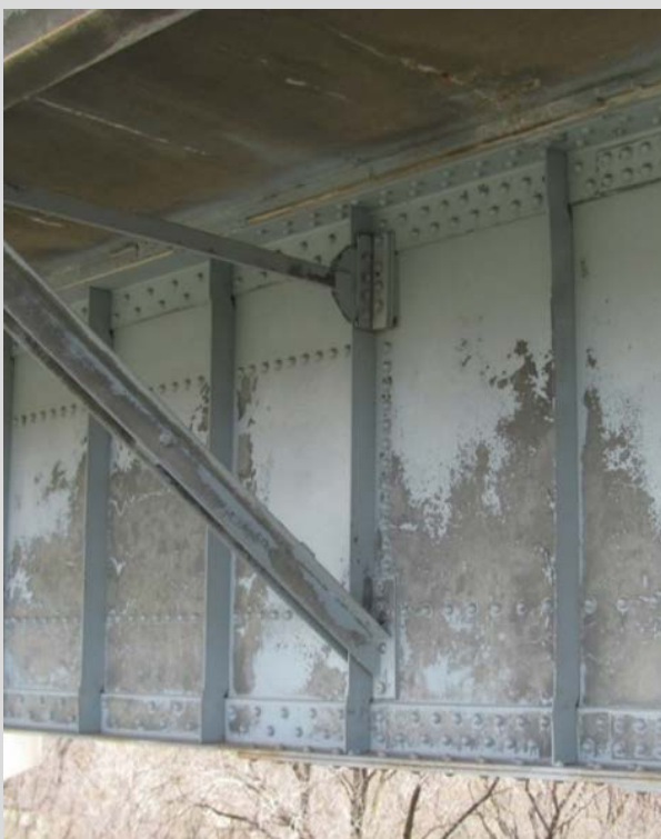
Condition State 3 Paint finish coat failure (primer coat remains intact)
