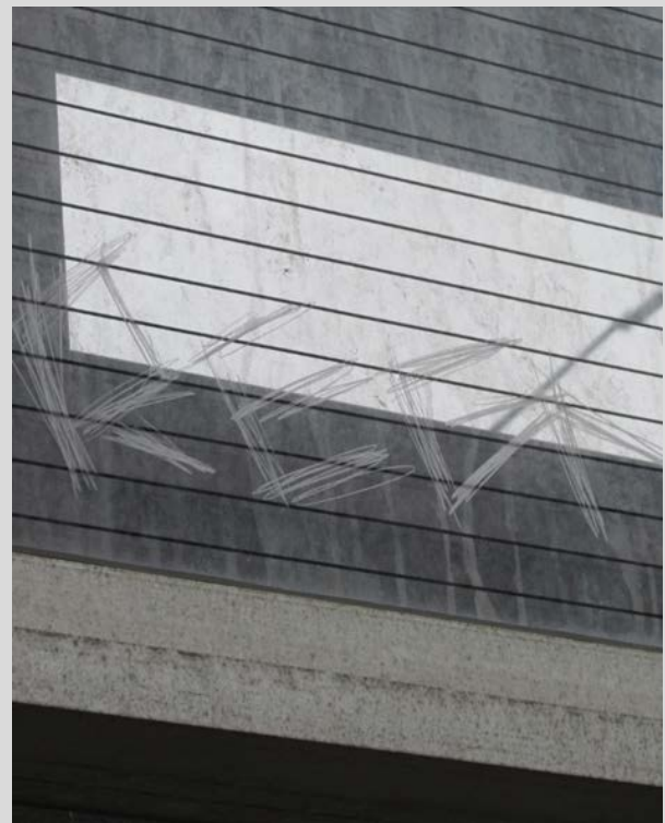
Condition State 2 Transparent Noise Barrier scratched by vandal.
