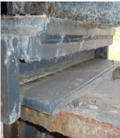
Scrape marks on a sliding plate hinge bearing indicate recent movement
