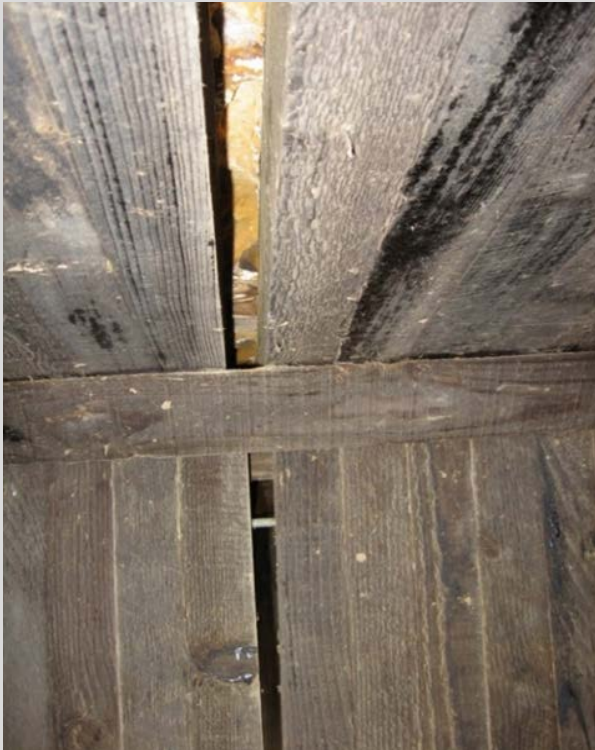
Condition State 2 Separation between timber members on a timber box culvert (no backfill infiltration)
