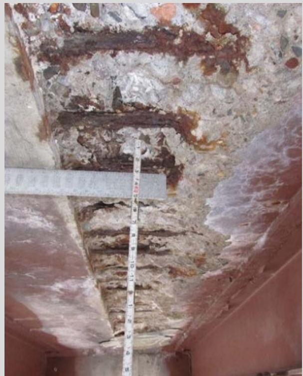
Condition State 4 Severe spalling (more than 3" deep) on the underside of a concrete deck
