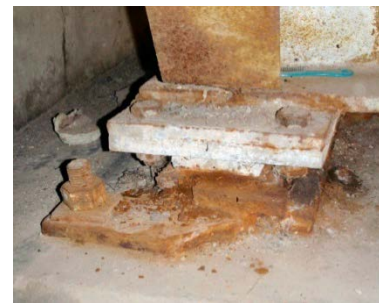
Corroded (possibly frozen) sliding plate bearing
