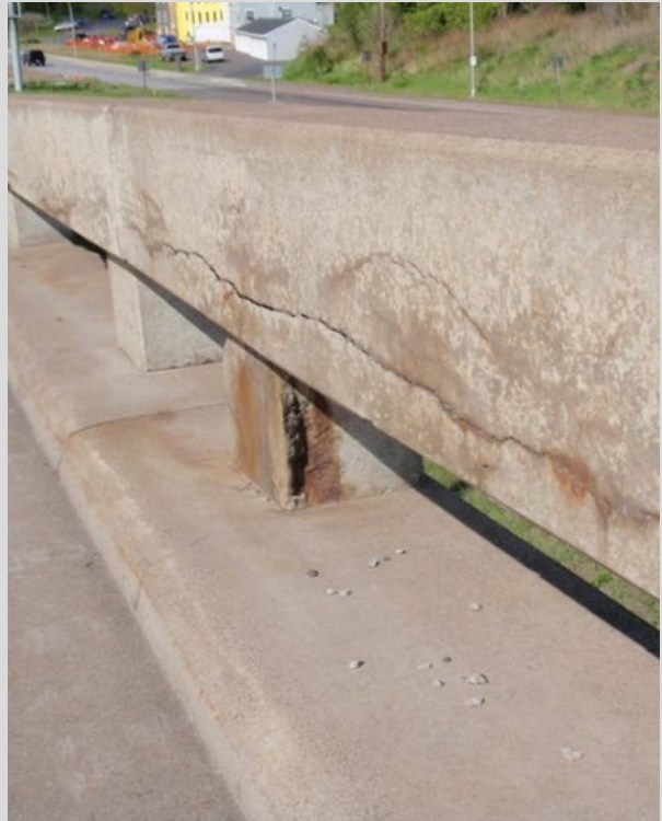
Condition State 3 Cracking, delamination, and rust staining on a concrete post & beam railing
