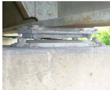
Uplift (gap) on a curved plate fixed bearing
