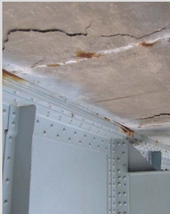
Condition State 4 Delaminated and loose concrete on the underside of a concrete deck (over traffic - safety hazard)
