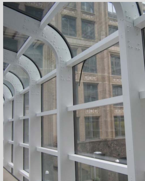
Condition State 2 Loose seal (no leakage) on an enclosed pedestrian skyway
