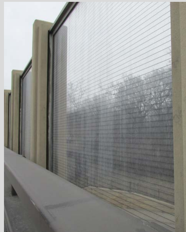
Condition State 1 Transparent Noise Barrier is dirty (no permanent loss of transparency)
