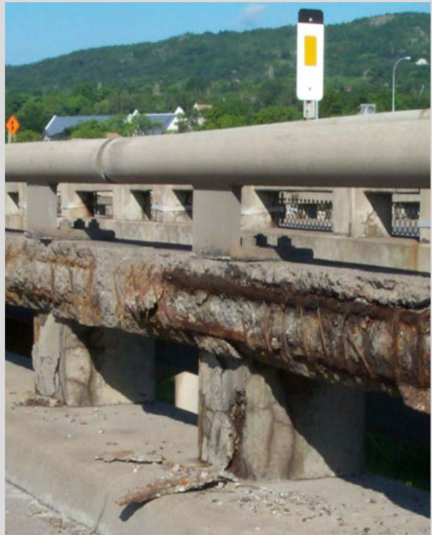
Condition State 4 Severe spalling on the concrete rail base of a combination railing
