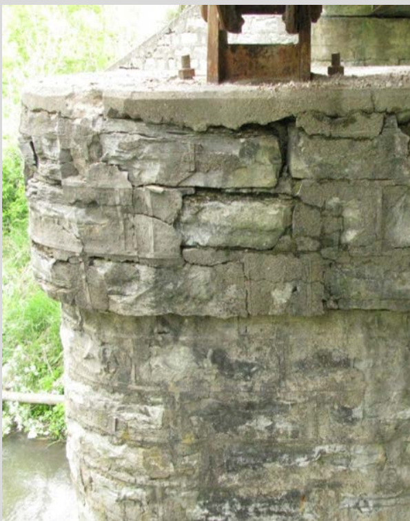
Condition State 4 Masonry pier wall severely deteriorated below a truss bearing
