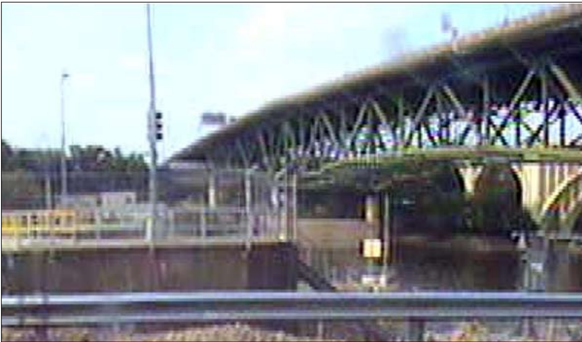
Figure 10. Close-up of first image of collapse sequence, captured by surveillance camera at 18:04:57. The south (near) end of the center span can be seen to have dropped from its position as shown in precollapse images (compare with figure 9).
